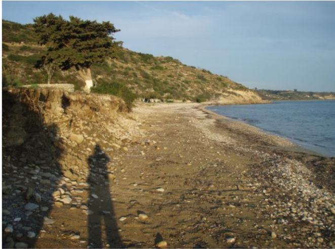
Figure 2.1: Erosion on Agia Barbara, 2008
